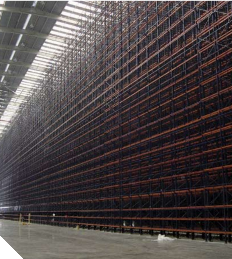
SafeStore, 35 meters high and 125 meters long installation in the lateral of a new automatic warehouse. The installation is made for Porcelanosa Group, a well known Spanish company within the ceramic world with headquarter in Villareal (Castellón).
