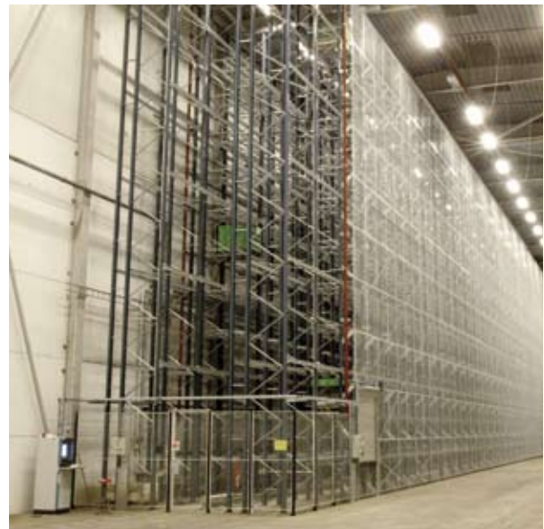
SafeStore combined with FlexiStore around an automated warehouse at Scania in Sibbhult, Sweden. The equipment is delivered by Constructor, Sweden. Axelent's hinge door with cylinder lock, see pages 18-20, has been chosen along with the mesh wall system.
